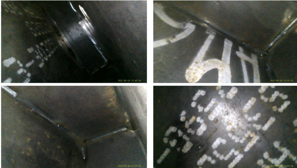
Figure 6.33: This figure shows a selection of endoscopic photos taken from the inside of the 4-cell-prototype before the coating process. The inner walls are covered in rust and writing from the construction of the prototype.
