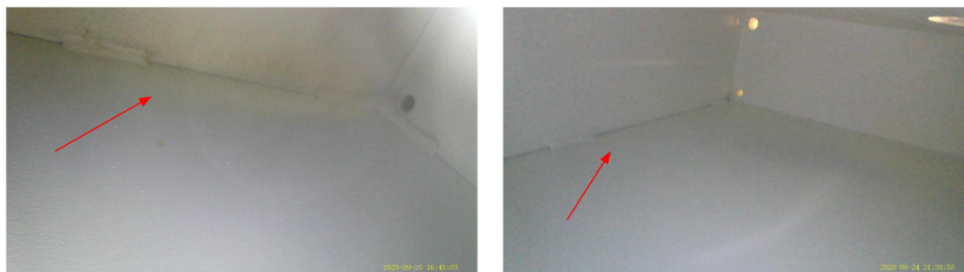
Figure 6.34: Left: A large yellow stain developed in the first layer of primer due to water in the pressurized air. Right: The following layers of primer and coating were able to fully cover this area.
