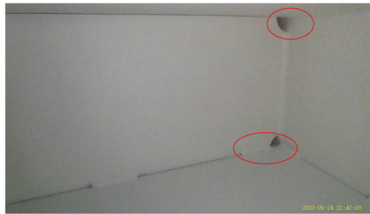
Figure 6.36: Some areas around weld seams and connecting holes between the cells show slight yellow discoloration in the final coating result. This is due to the primer showing low adherence to the seams and not being able to fully cover the connecting holes with primer.
