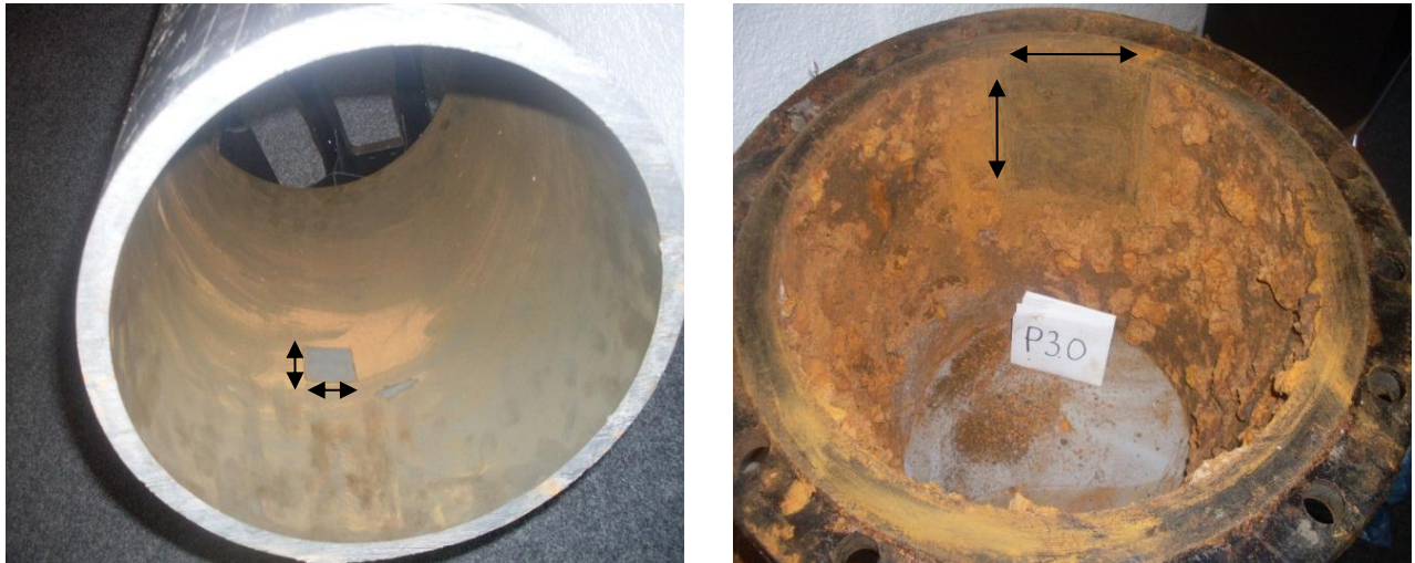
Figure (8-17) Corroded surface scales on the pipe
