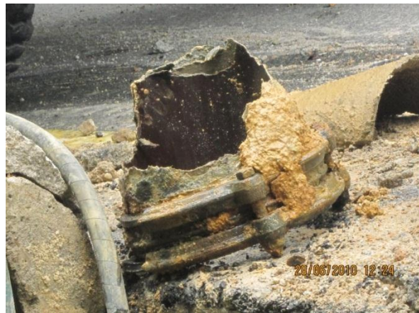
Joint failure of AC pipe
