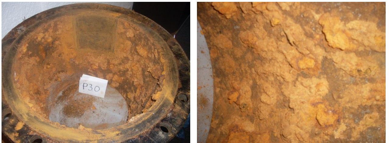
Figure (8-18) Corroded surface scales on the iron pipe
