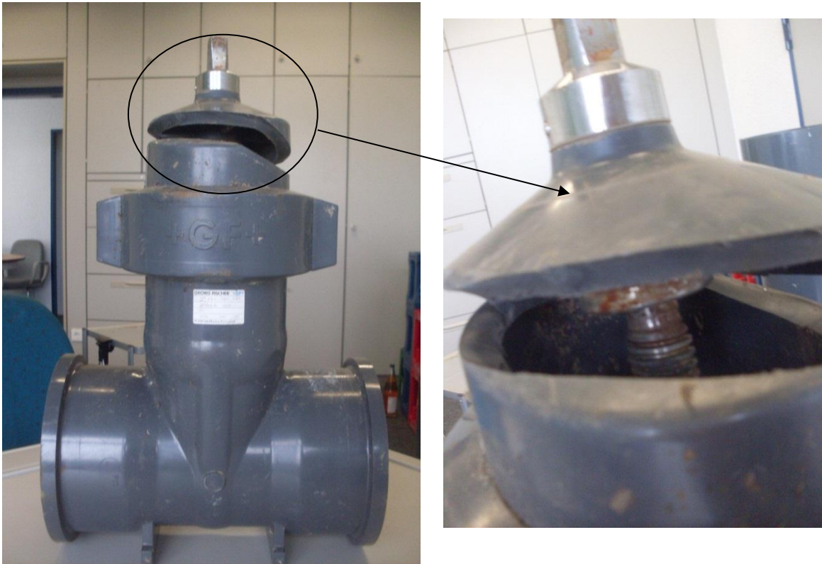
Figure (8-15) Failure case (H-3) for UPVC pipe valve failure
