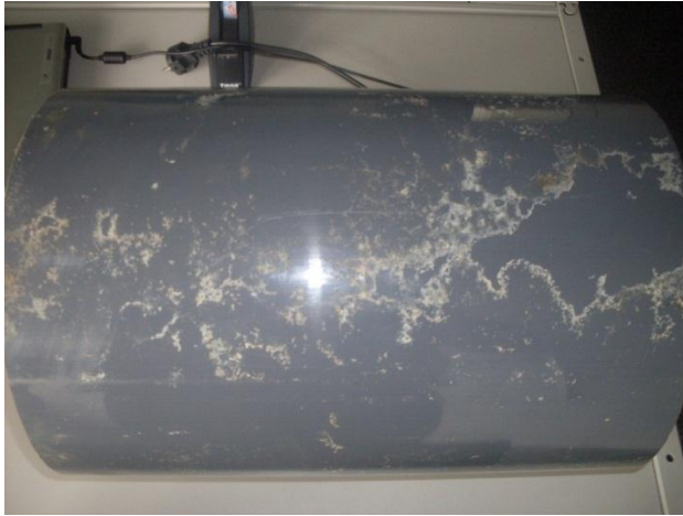
Figure (8-22) Bottom view of the UPVC pipe after 30 years installation.
