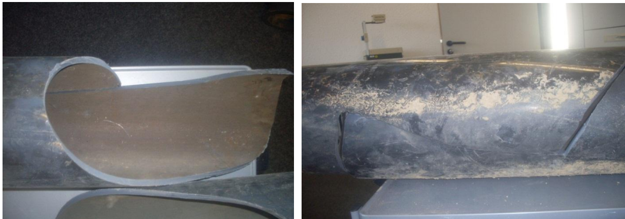
Figure (8-14) Failure case (H-2) for UPVC pipe failure
