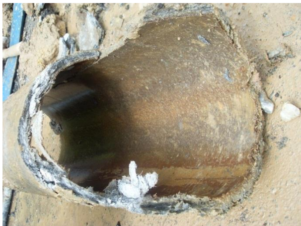
AC pipe failure
