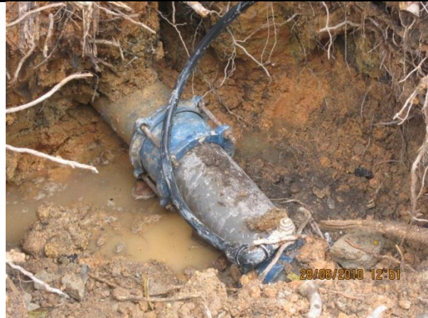
Failure of AC pipe surrounding by roots
