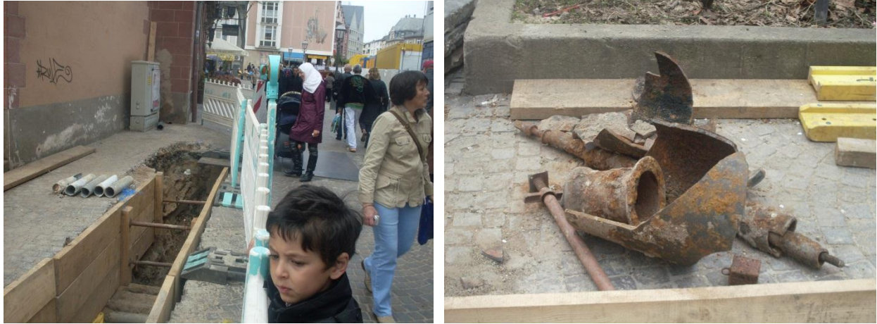
Figure (9-36) sample for pipe failure disruption in the center of Frankfurt am Main city
