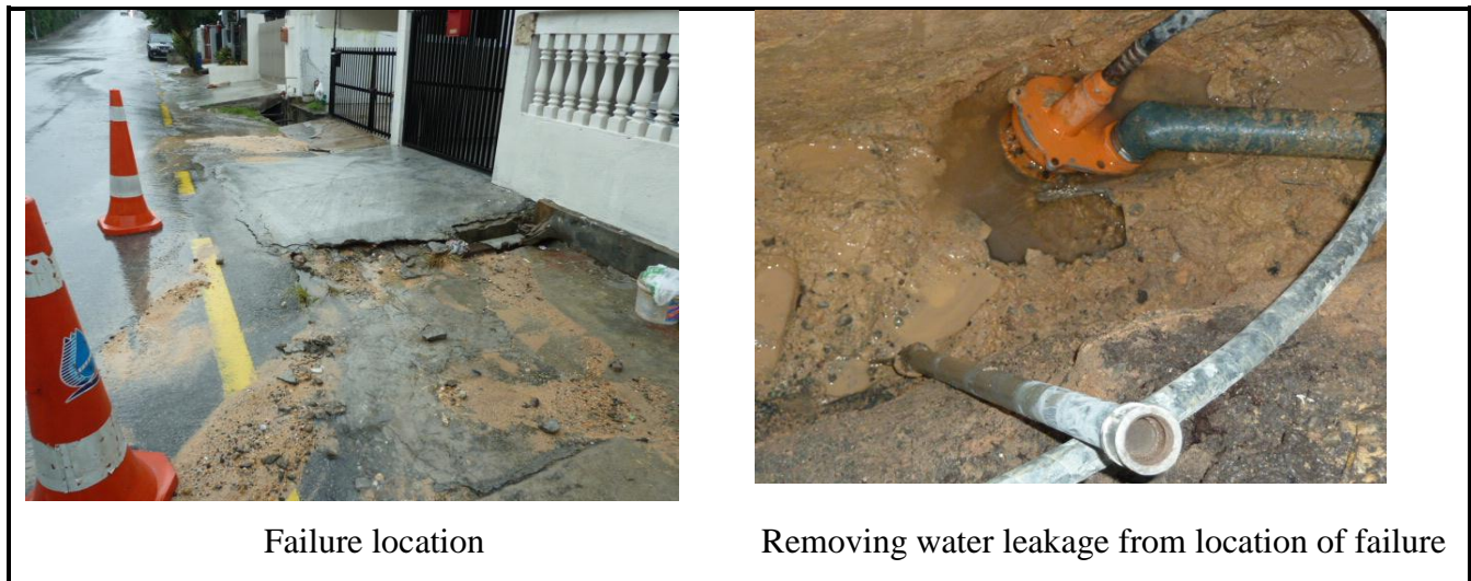
Figure (4-3) Pipe failure samples from Kuala Lumpur
