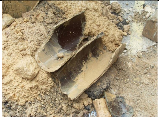
Failurte due to high water pressure
