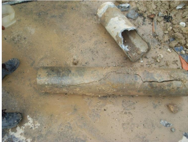
Figure (7-15) View of AC pipe Sample as received condition after failure
