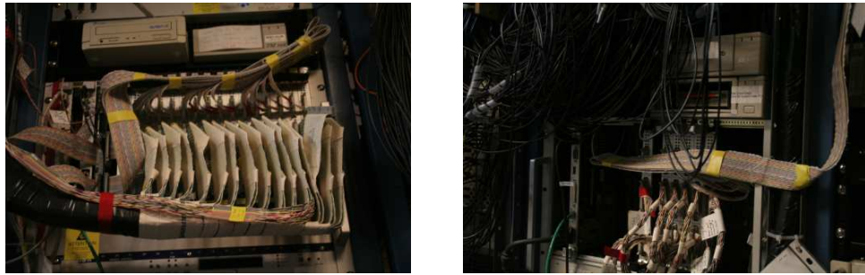
Figure 2.13: Some components of the muon DAQ. Left: one of the AMANDA crates - right: the DMADs, discriminator and adders which compose the trigger logic. Both are located in the Martin A. Pomeranz building.
