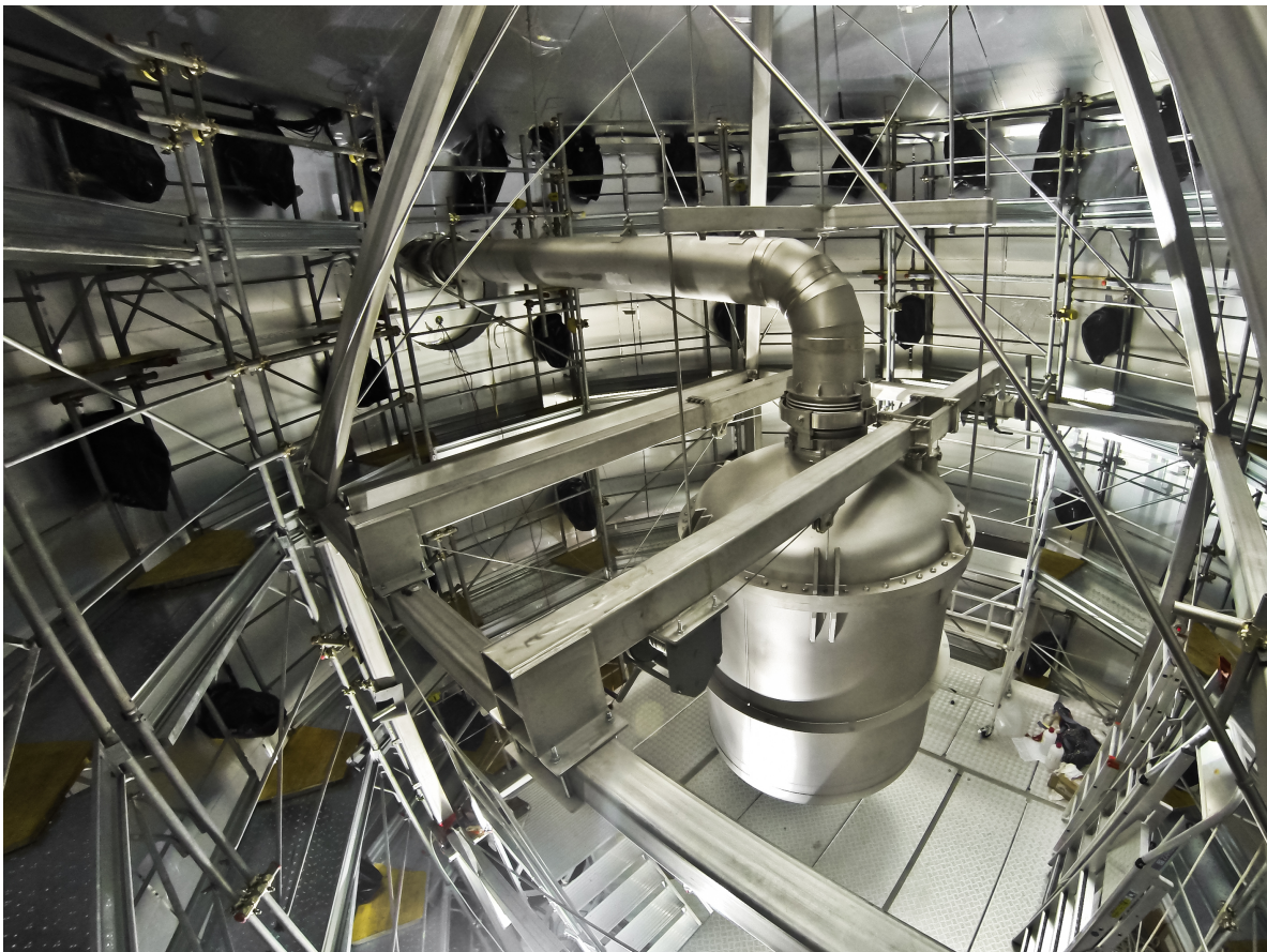
Figure 7.2 – A view inside the active muon veto of XENON1T: The cryostat in where the TPC will be mounted is already installed. The scaffold on the site of the walls will be removed as well as the black protection layers of the veto PMTs [44].
