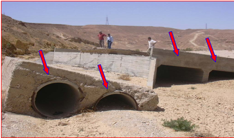
Photo (1) the highway and bridge in Wadi Water were destroyed by a flash flood
