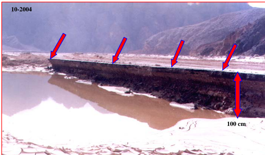
Photo (2) the flash flood attacked the road and eroded it vertically of about 100 cm
