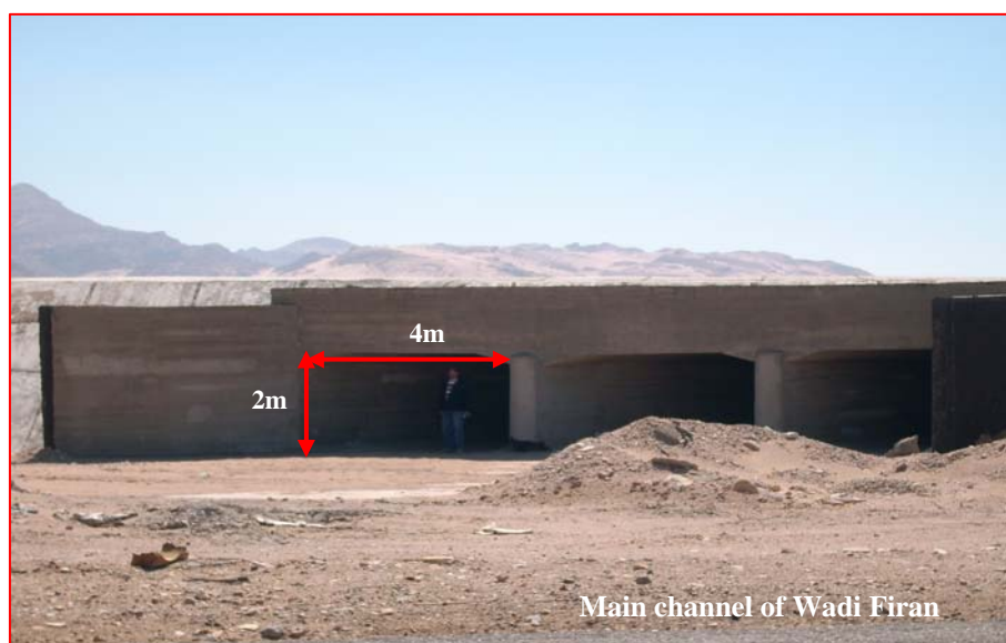
Photo (5-7) Construction of diversion for the main channel of Wadi Firan above the delta
