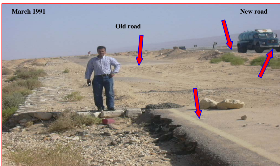
Photo (3) the highway Suez- Sharm El-Sheikh was destroyed by a flash flood of Wadi El-Aawag
